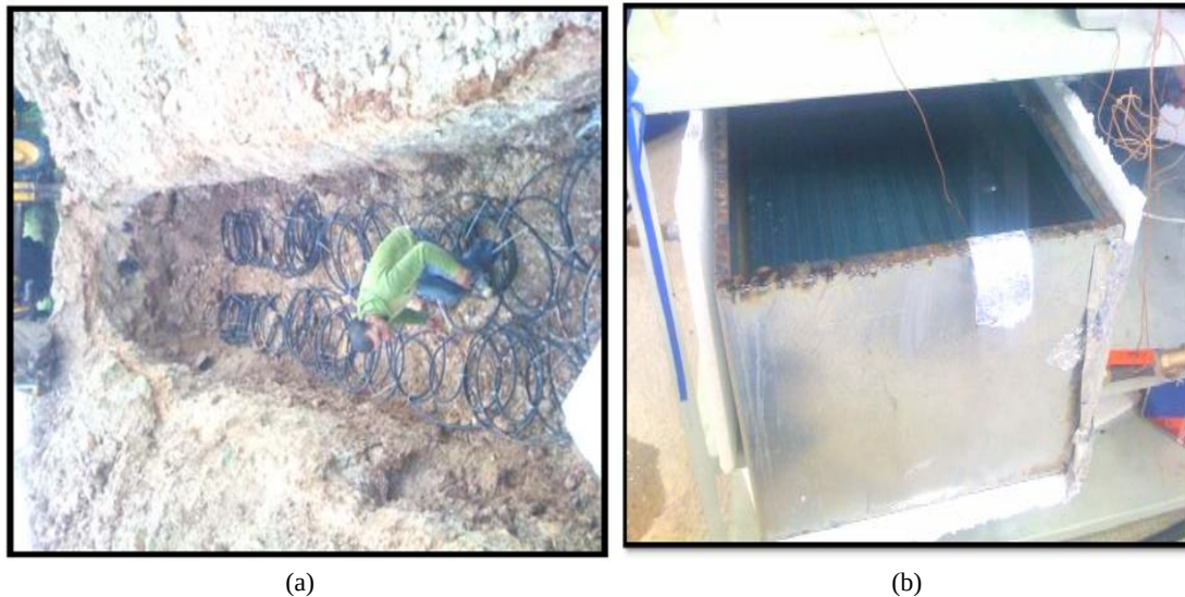
Figure 1a: Installed system loops Figure 1b condensing unit inside the loop
