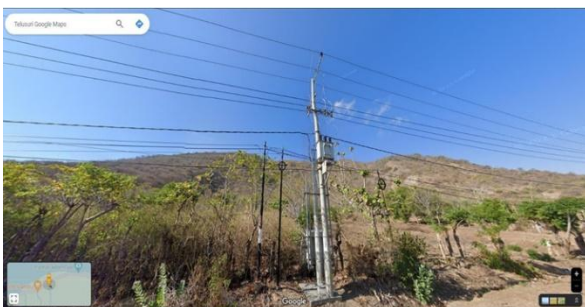
Figure 2.1. AL114 Substation on the Tambak Sari Feeder (Source: Google Maps)
