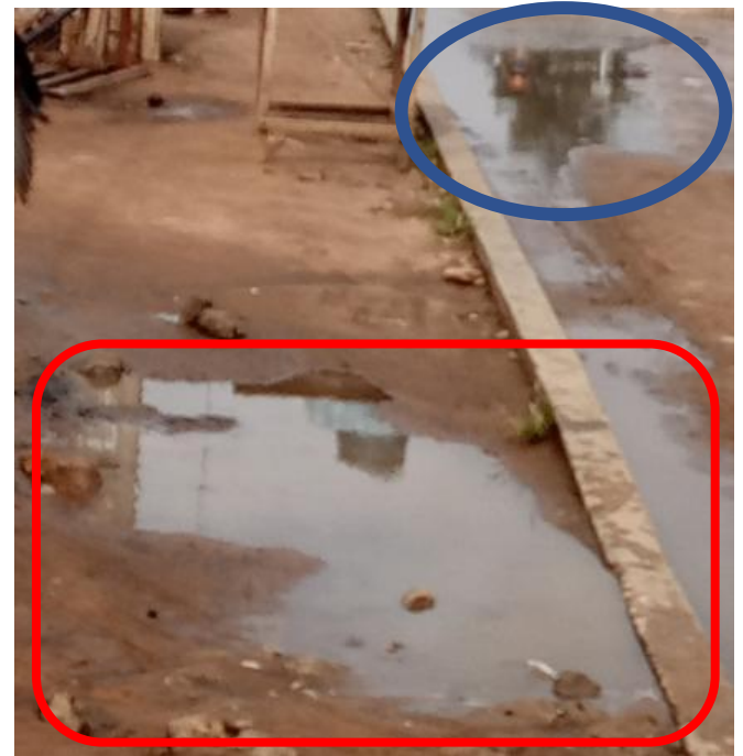
Figure3: Puddles on the road and sidewalk after rain
