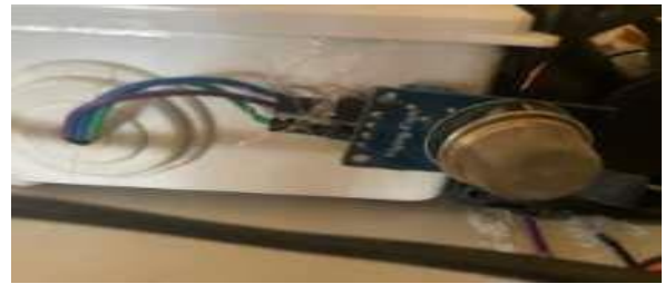
Figure 10: Gas detector connection
